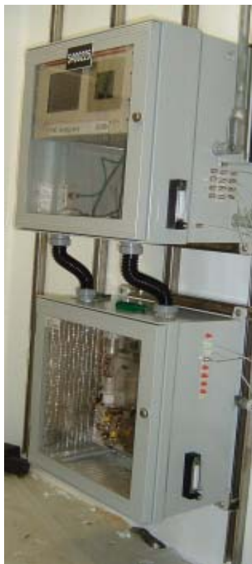
Model 301 C (above) in instrumentation housing at a Chlorine plant measuring H_2 , O_2 , N_2 & CO_2 . TCD with hastelloy valves & fittings. The Analyzer and oven (lower enclosure) are purged to keep corrosive atmosphere from Analyzer.
