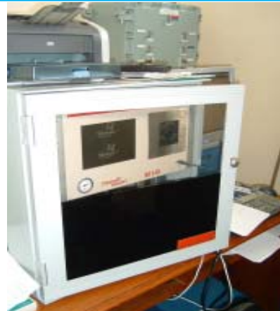
301C installed at a natural gas odorant facility for measuring THT & TBM on-line.
