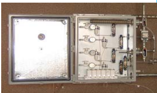
Sampling system for wet chlorine (above) has teflon valves and multipoint. sampling system is heated to prevent condensation. The sampling system valves are controlled by air actuated valves in the 301C.
