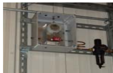
Sampling system for moisture removal and measurement of S cpds at ppb levels.
