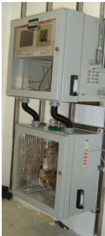
Model 301 C (above) in instrumentation housing at a Chlorine plant measuring H 2 , O 2 , N 2 & CO 2 . TCD with hastelloy valves & fittings. The Analyzer and oven (lower enclosure) are purged to keep corrosive atmosphere from Analyzer.
