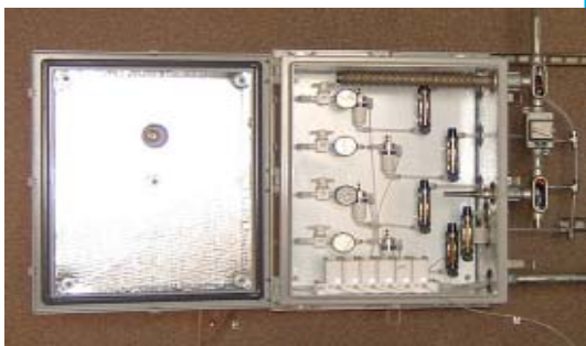
Sampling system for wet chlorine (above) has teflon valves and multipoint. sampling system is heated to prevent condensation. The sampling system valves are controlled by air actuated valves in the 301C.
